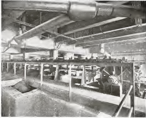
Coal Conveyor—The Wanamaker Power House, Philadelphia, Pa.
